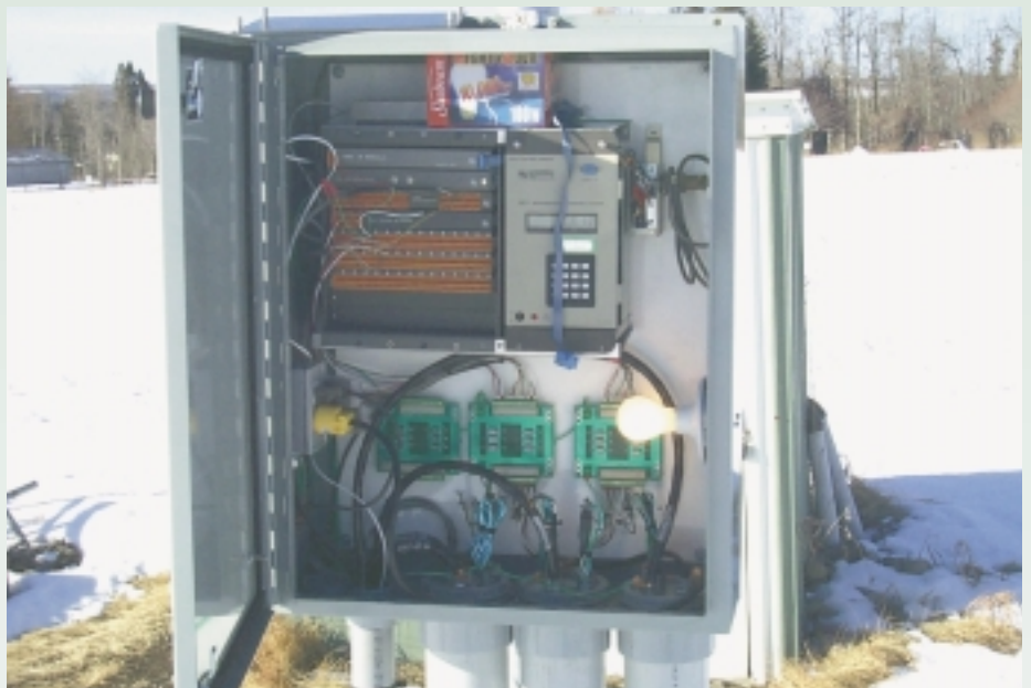
Figure 3: Remote Sensor Installation (image courtesy: D. Puurveen, Edmonton, Canada).
